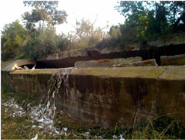
Tramo del colector colapsado
